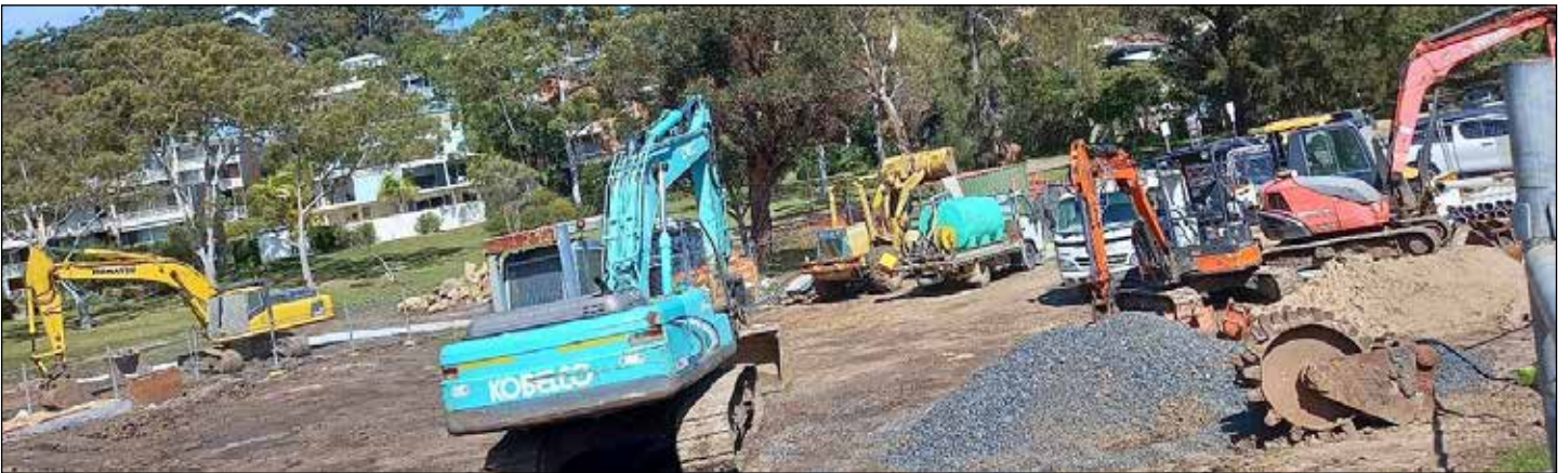
Council continues to work on the drainage problem.
