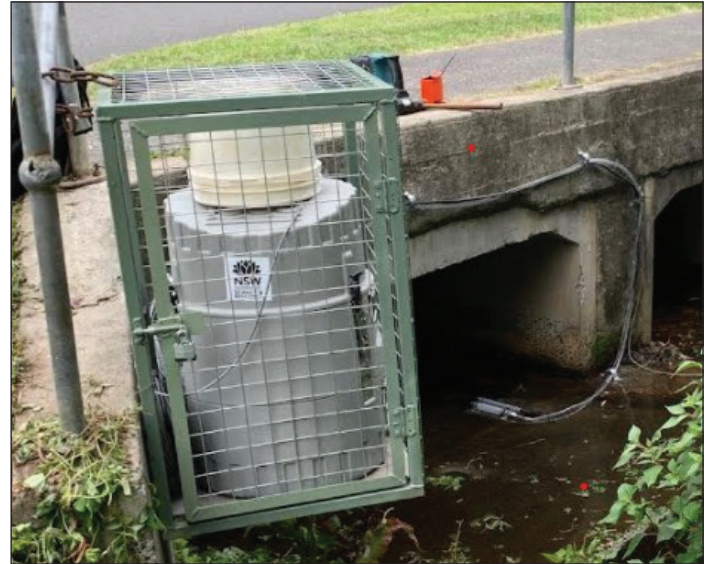
Figure 2: Auto-sampler unit above and below water on Round Drive
